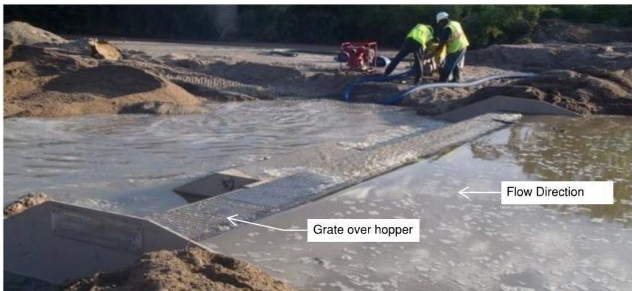
Figure 6: Image of bedload collector being installed. Note the open grate where bedload will fall into the trough below (Streamside 2020).
